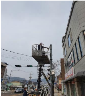
Power supply line connection
