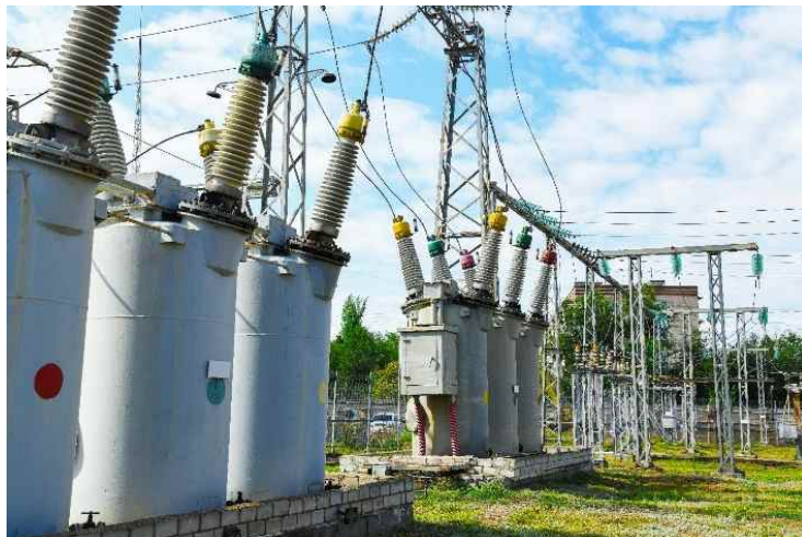
Oil Circuit Breaker
